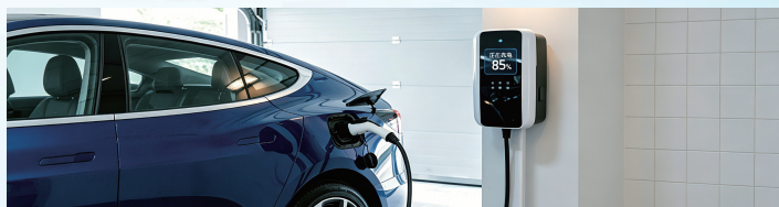
EV Charger Ready Drive for free
