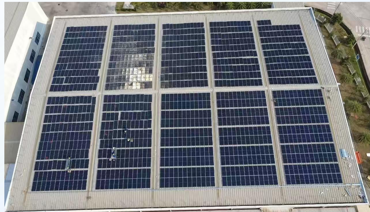
YAHU (THAILAND) 0.75 MW
